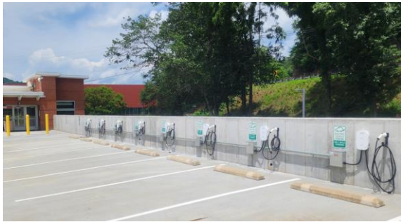
New EV Chargers at Parking Deck
