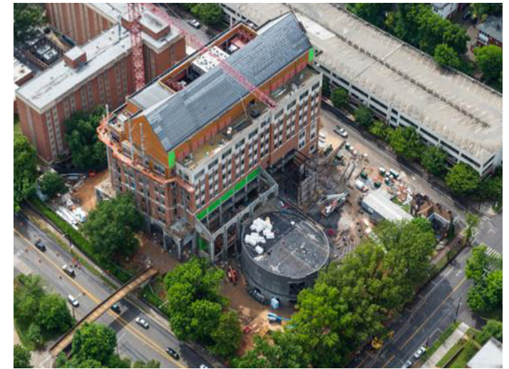
Above: On the UT Strong Hall Laboratory, Proposed Senior Superintendent, Aaron Isbill, partnered with the designer and owner during a 16-month pre-construction process that included extensive constructability review.
