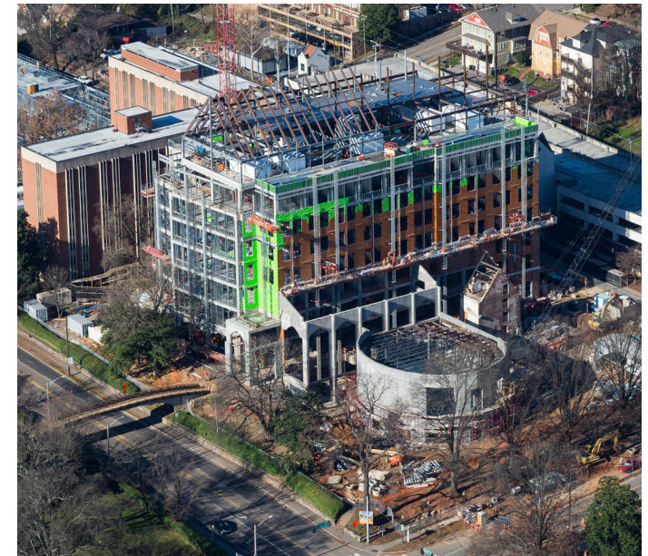
Image above: The Strong Hall Laboratory for the University of Tennessee. This project is coordinated entirely in BIM by our team, and features extensive laboratory spaces for chemistry, biology, as well as storage and habitat for live animals.
