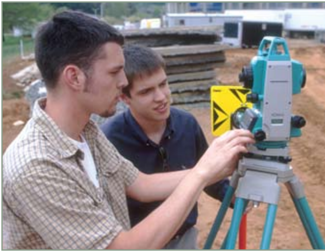
Kimmel & Associates' pledge benefits students such as the Western students pictured here at a construction site on campus.
