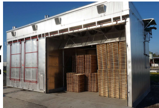
Fully loaded drying kiln
